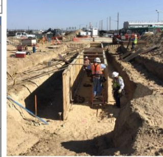
Formwork for Stormwater Planter west side of Brighton, south of 48th and Brighton intersection
