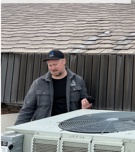
Matt assesses a rooftop unit and with input from facility staff, determines remaining design life.
