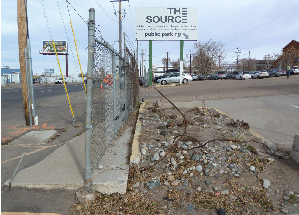
Twisted rebar at the entrance contribute to a sense of a general lack of maintenance
