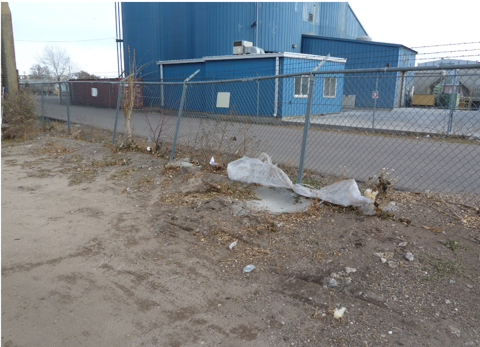
The fence at the rear of the property is dilapidated and collects trash and vegetation
