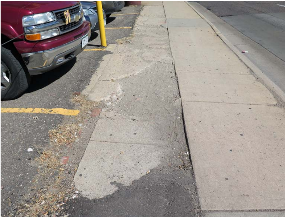
A sidewalk in degraded condition along Colfax
