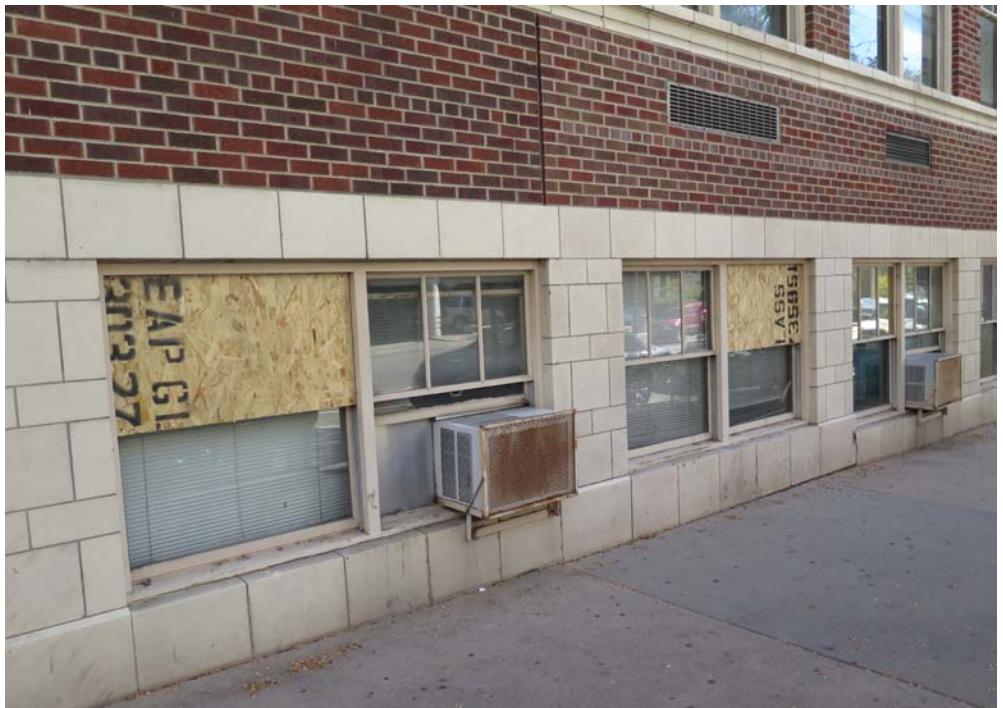
Broken windows at Emily Griffith property
