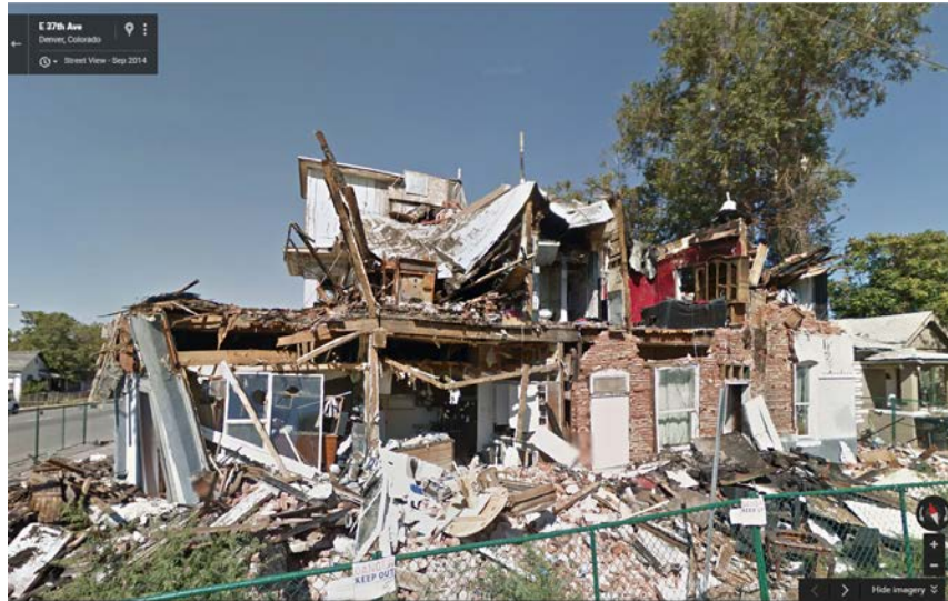
The ruins of the former structure as it appeared in August, 2014. Source: Google Street View
