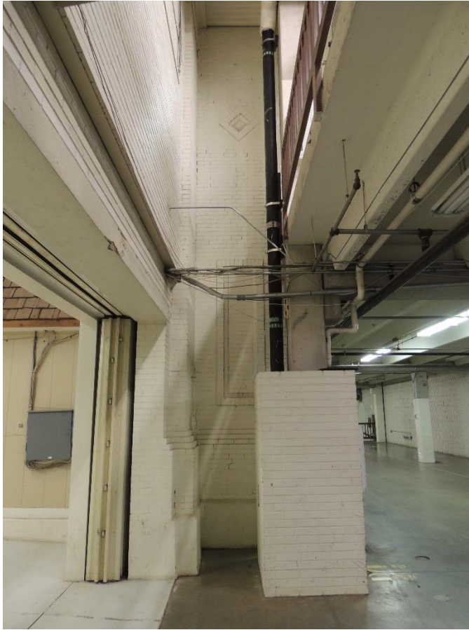
Figure 32. Widened entry and pocket door on the north side of the Stadium Arena, opening into Stadium Hall, showing the space between the original building and the addition. Photographed February 9, 2016, Dianna Litvak.
