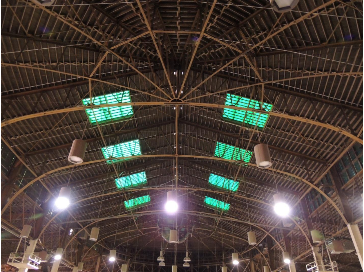
Figure 12. Steel roof trusses and interior roof structure of the Stadium Arena. Photographed February 9, 2016, Dianna Litvak.
