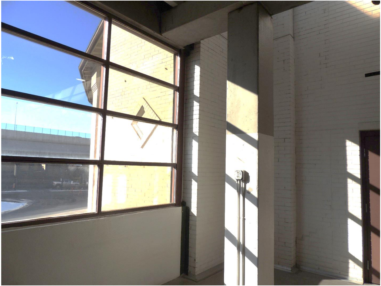
Figure 31. Stadium Hall exterior wall, shown touching the Stadium Arena's east end, upper level. Photographed February 9, 2016, Dianna Litvak.
