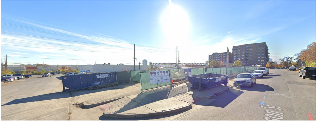
Current lot under construction across the street on North Jason Street, looking southeast.
