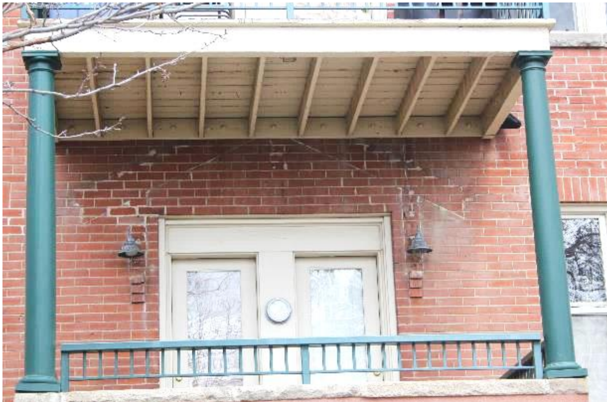
Figure 27. Detail of west wing 1 st floor porch. Ghost of original gabled entry canopy is visible with projecting corbeled brick supports remaining in place. Photograph by Paul Cloyd, February, 2018.
