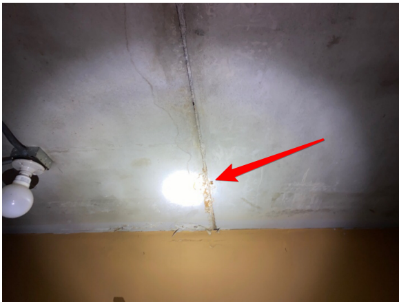
Visible leaking on ceiling
