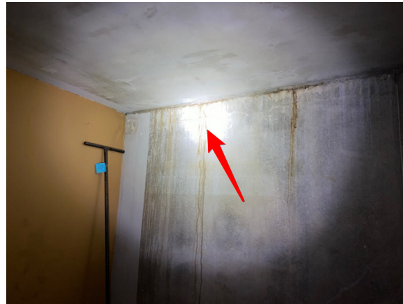
Visible leaking on wall
