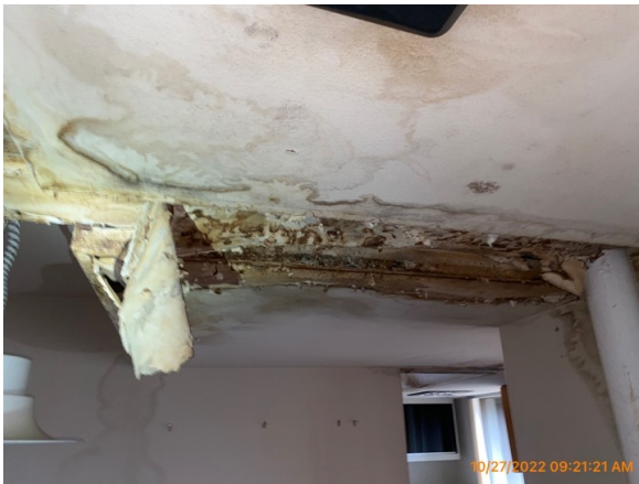
Leak at concrete seam
