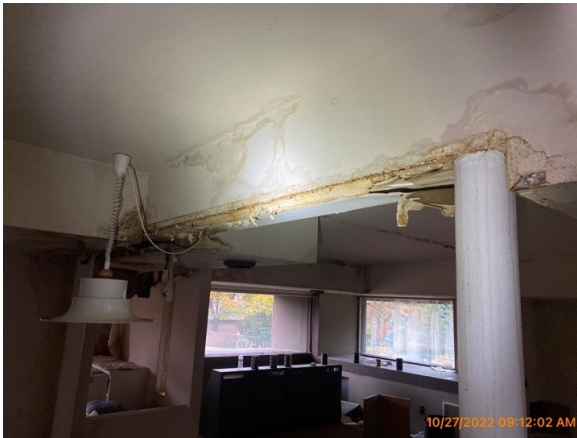
Framed in support beam with signs of leaks
