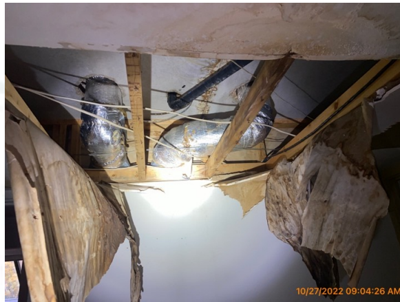
Drop down ceiling with damage and microbial growth
