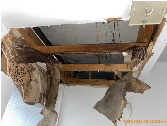
Framed in drop down ceiling with signs of leaks
