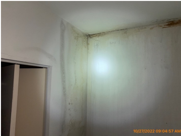
Microbial growth and leak at wall
