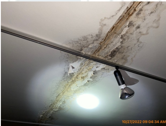
Leak at concrete seam
