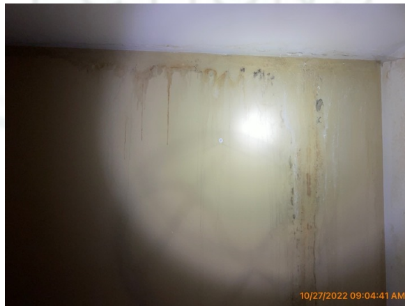
Microbial growth and leak at wall
