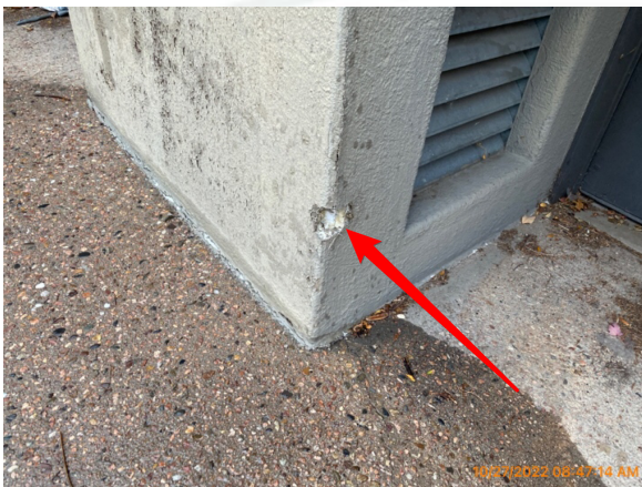
Damage at corner
