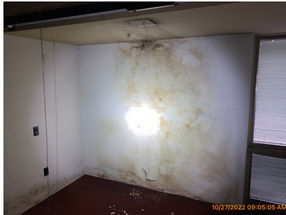
Microbial growth and leak at wall
