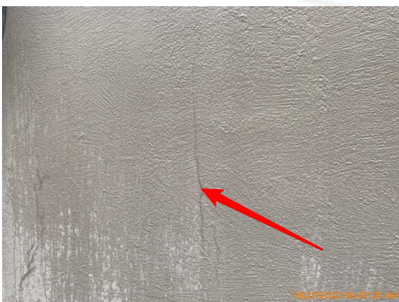
Cracks visible in stucco
