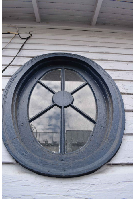
6. Oval bullseye window on the north wall. Photographer: Thomas H. Simmons. Date: August 2023. View south.
