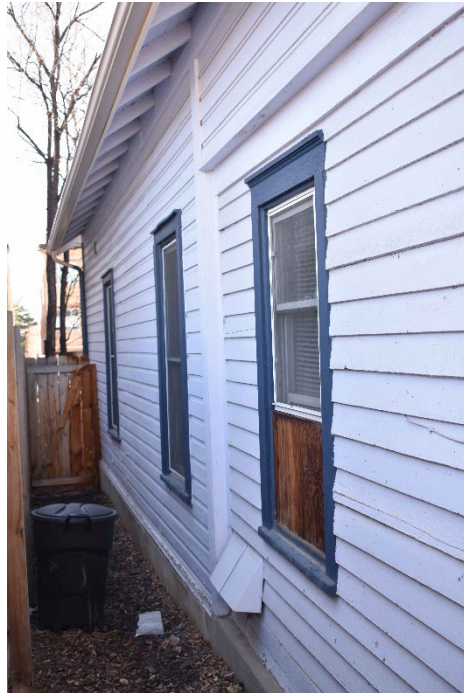
9. South wall from the backyard. Photographer: Thomas H. Simmons. Date: March 2024. View west-northwest.
