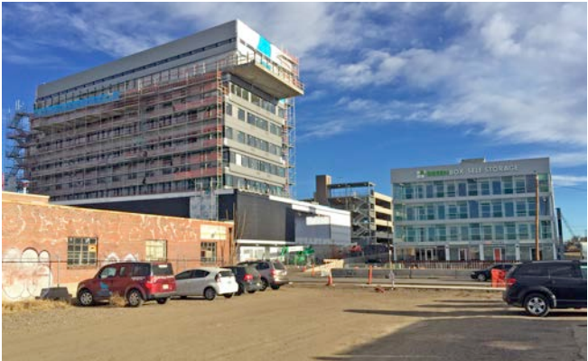
The Source Hotel (left) is currently under construction adjacent to the GreenBox mini-storage facility on Brighton Blvd. on the northwest side of the A Line commuter rail. This area would be included within both the DO-7 and IO-1 overlay districts.
