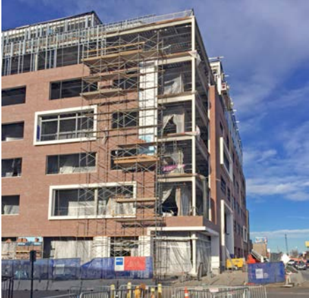
The multi-story commercial Catalyst development is under construction at 35 th and Brighton Blvd. This area would be included within both the DO-7 and IO-1 overlay districts.
