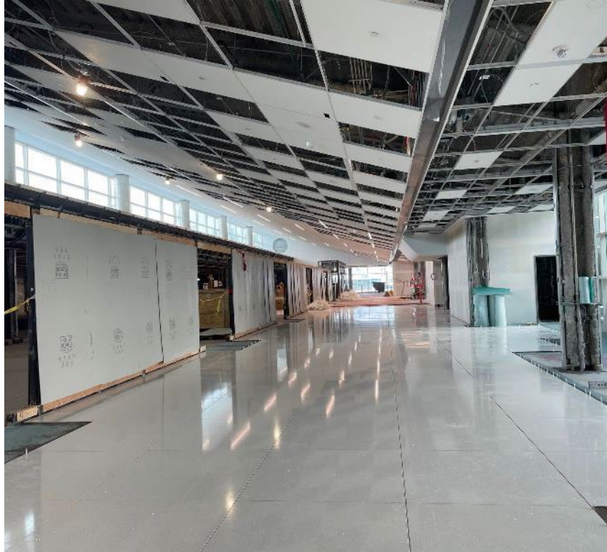
Progress of the East Security Checkpoint shows new flooring that was recently installed
