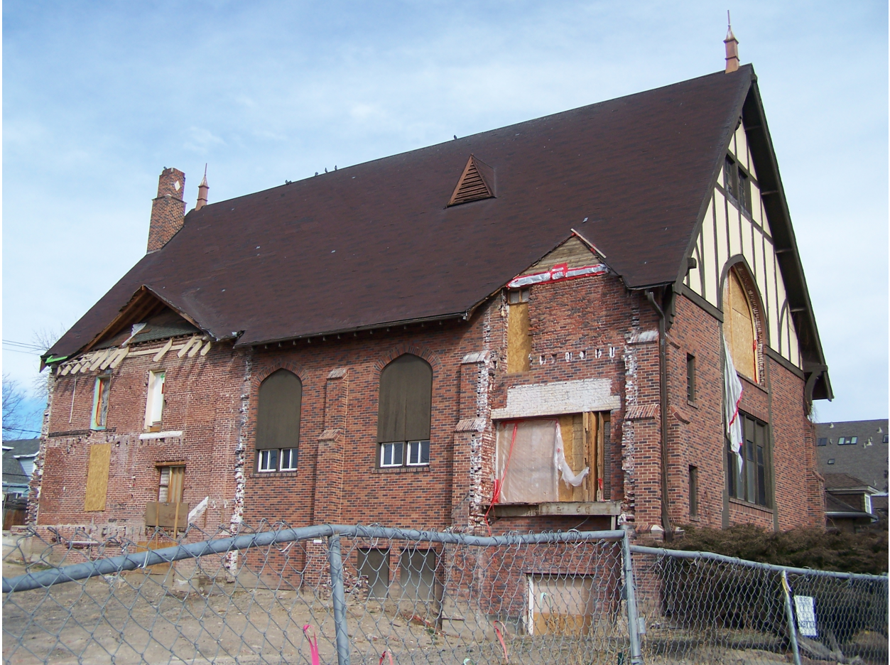
Photograph 4. The South façade, with the later additions to the church (including the 1934 vestibule) now demolished.
