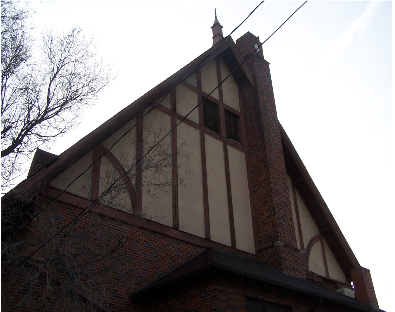
Photograph 6. A closer view of the West façade, showing the detailing on the chimney and finial on the roof.
