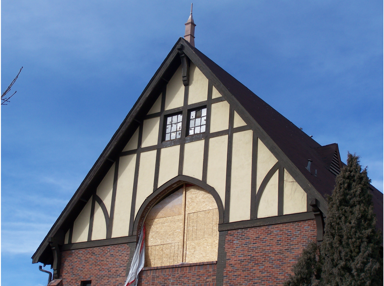
Photograph 3. East façade, showing the decorative brackets at the eaves of the roof.
