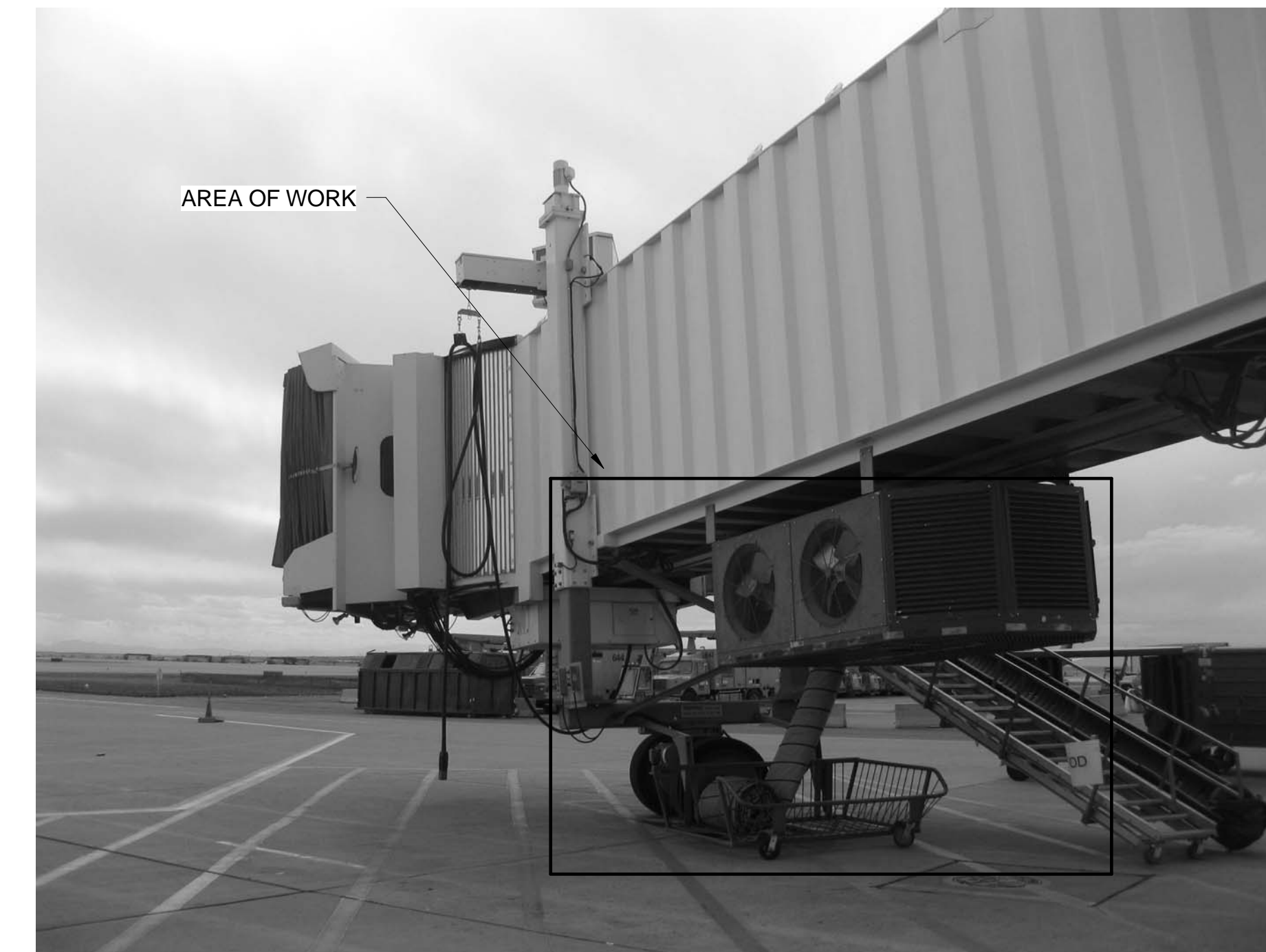
1 M0.01 TYPICAL EXISTING PCA UNIT INSTALLATION NOT TO SCALE
