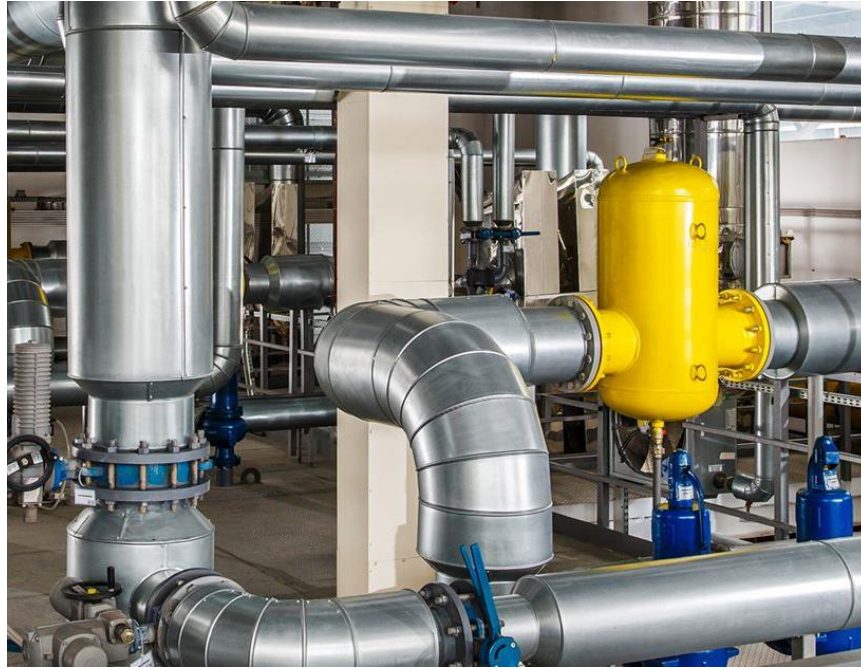
Central System with Tank
