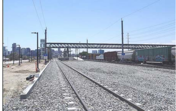
Recently constructed pedestrian bridge at the 41 st and Fox Station platform construction site (Source: RTD)
