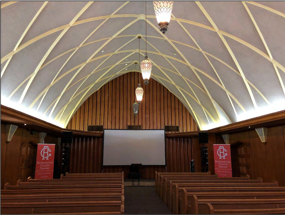
7. Interior of chapel. Note decorative plastered ceiling and wood paneling. View north, March 2020.
