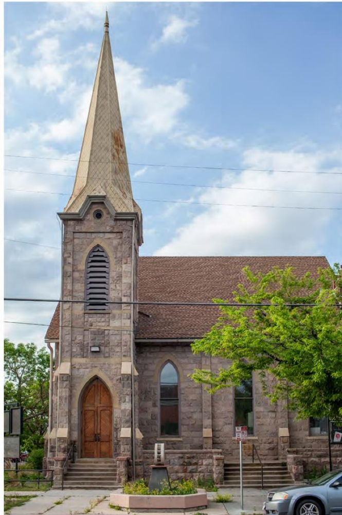
South elevation of original chapel showing the bell tower, lancet windows and doors, stonework, and original metal shingling.
