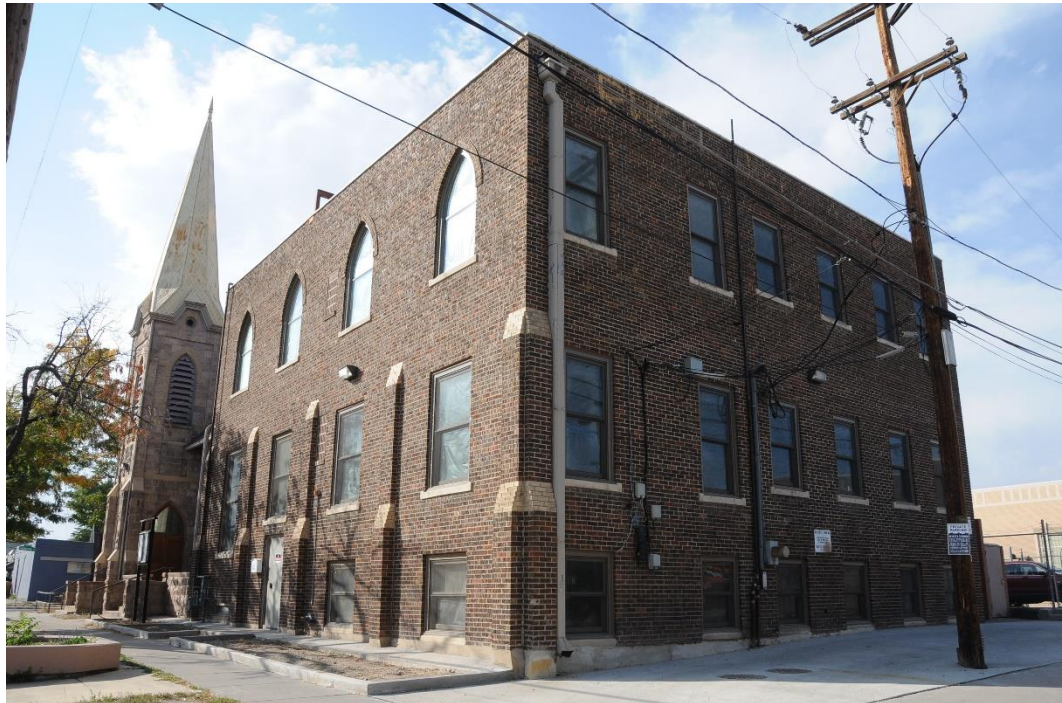
Southeast façade of Smith's Chapel and 1923 addition. Photo by Shannon Schaefer Stage, Oct. 2020
