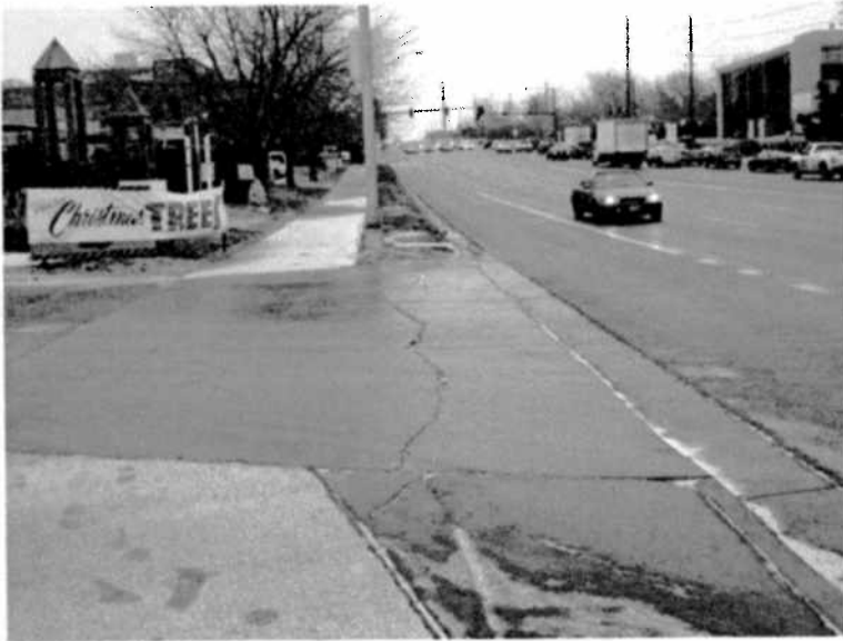
Figure 2-1: Substandard curb cuts and cracked/uneven surfaces for pedestrians
