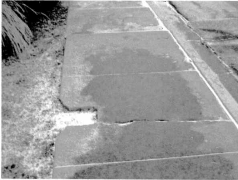
Figure 2-3: Deterioration/lack of site sidewalks/pedestrian areas
