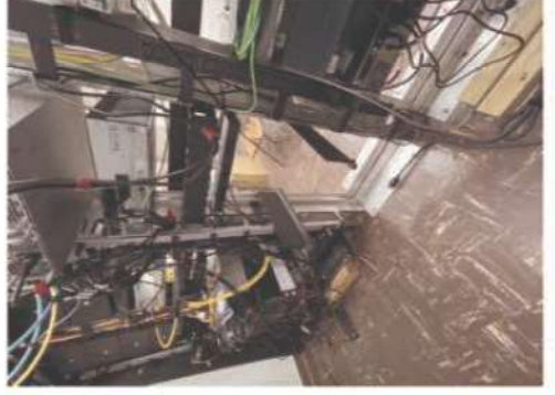
PDU for DAS/Verizon equipment
