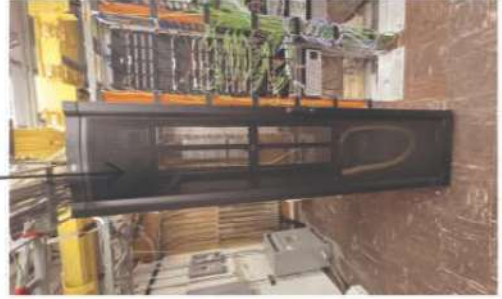
Cabinet for DAS/Verizon equipment
