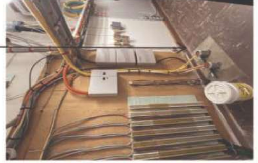
Unknown riser leading to 4th floor
