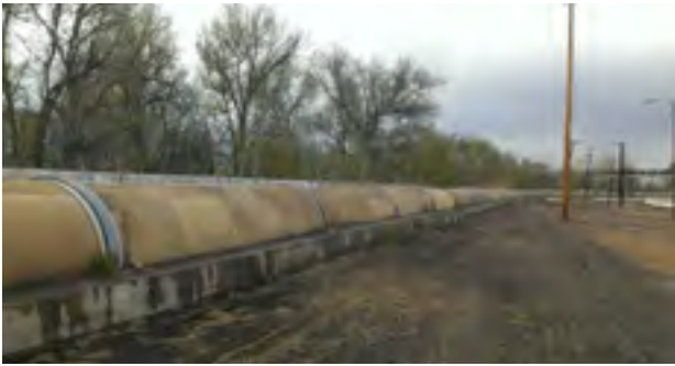
The Delgany Interceptor sanitary sewer lines run for almost 25 miles and are above ground along the NWC river frontage, creating a barrier between the NWC and the South Platte River.
