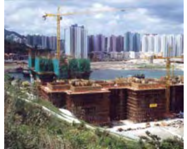
Dramatic growth in many places throughout the world will impact how Downtown Denver evolves. Cities like Hong Kong, China (above), will be in direct competition with Denver for natural resources, building materials and intellectual capital in the coming years.
