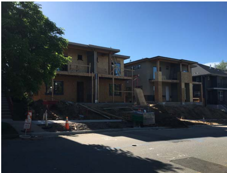
Two duplexes are under construction due west of the subject site, across the alley and facing Jackson Street.
