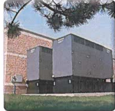
Figure 12. Backup Power Generators
