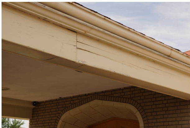
4034: Split wood elements
