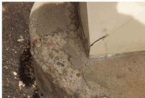
4035: Broken terra cotta, spalled concrete
