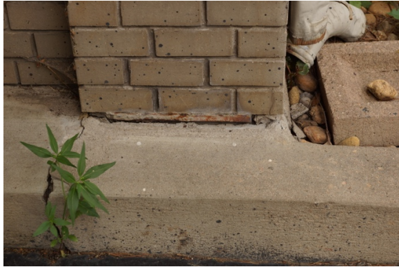
4020: Concrete cracked, mortar loss
