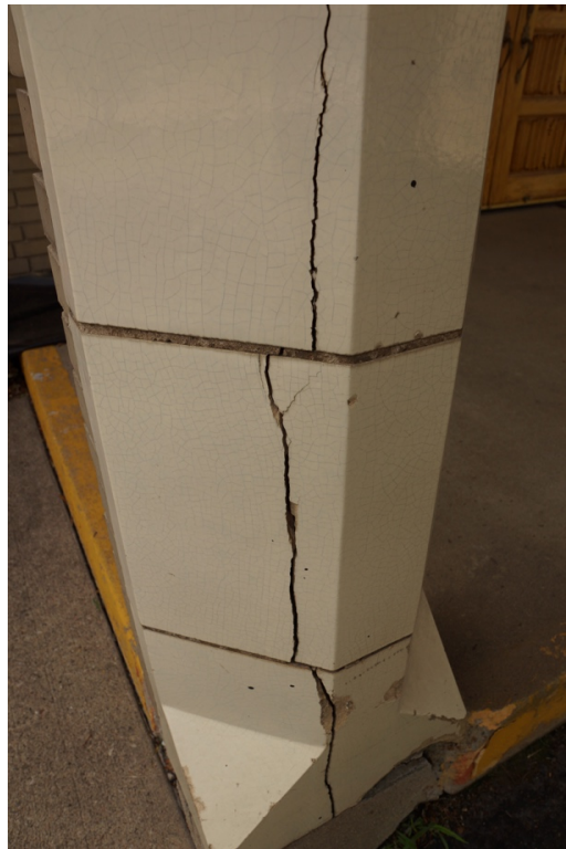
4049: Terra cotta damage
