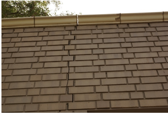
4053: Structural crack in brick wall
