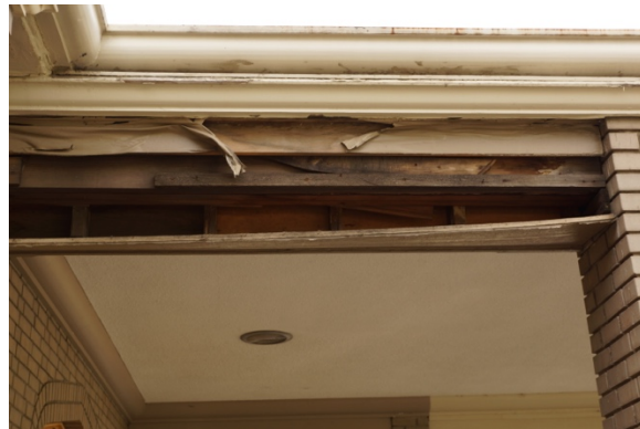
4023: Porte cochere prevalent damage
