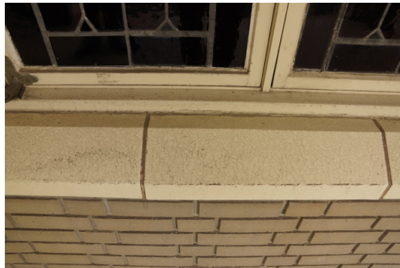
4047: Terra cotta damage
