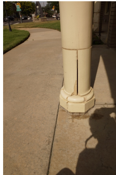
4041: Column base has typical terra cotta edge loss
