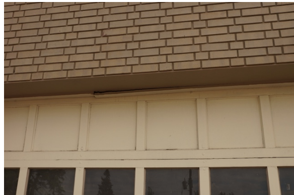
4029: Damage at head
