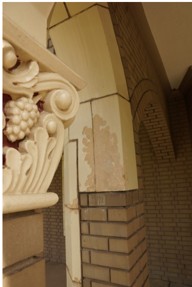
4042: Terra cotta glazing loss
