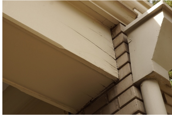
4021: Porte cochere prevalent damage
