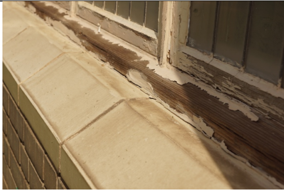
4038: Paint loss and rot
