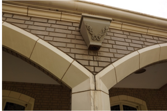
4045: Downspout is gone
