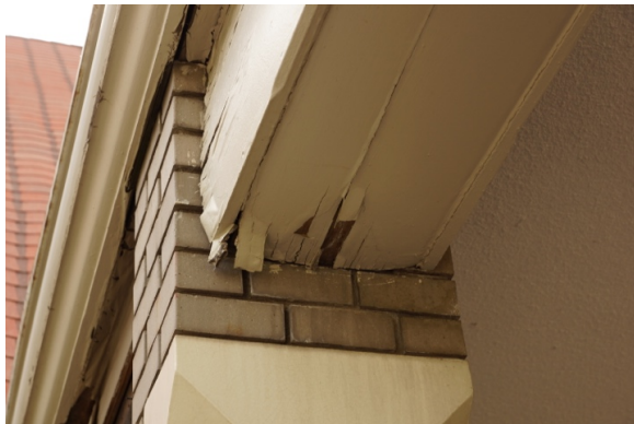
4022: Porte cochere prevalent damage
