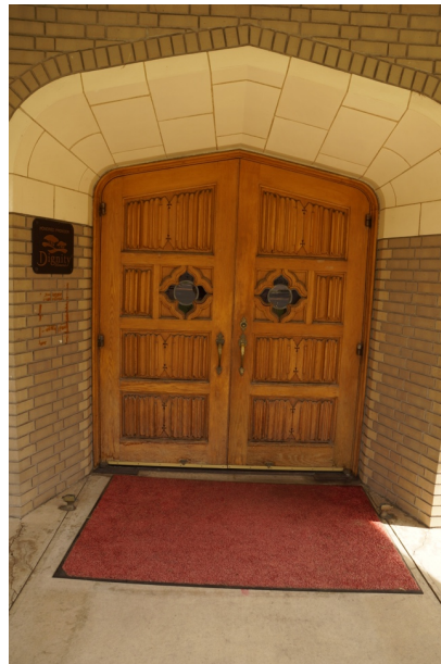
4043: Terra cotta, typical issues
