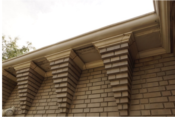
4051: Note damage between corbels at soffit
