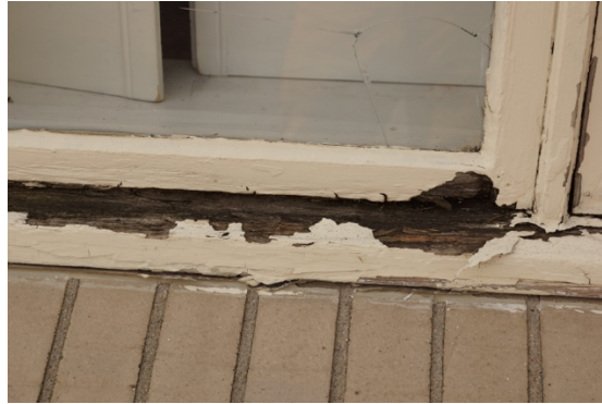
4033: Window deterioration, sill rot
