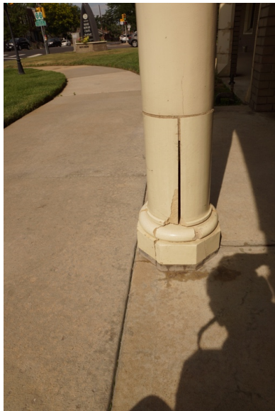
4040: Terracotta—mortar loss at column
