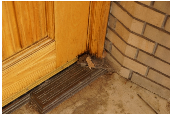
4037: Moisture uptake at entry door
