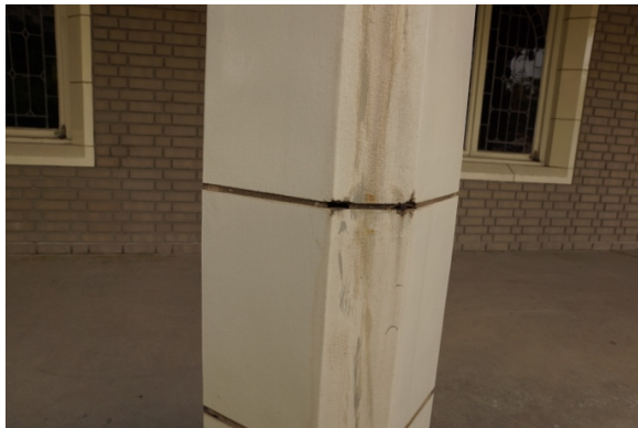
4046: Terra cotta damage
