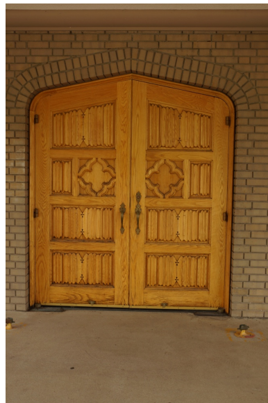
4019: Entry door water damage along lower edge
