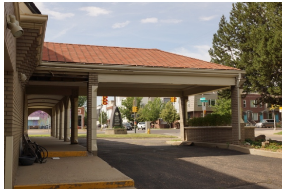
4025: Porte cochere prevalent damage
