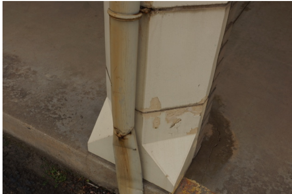
4016: Terra cotta damage
