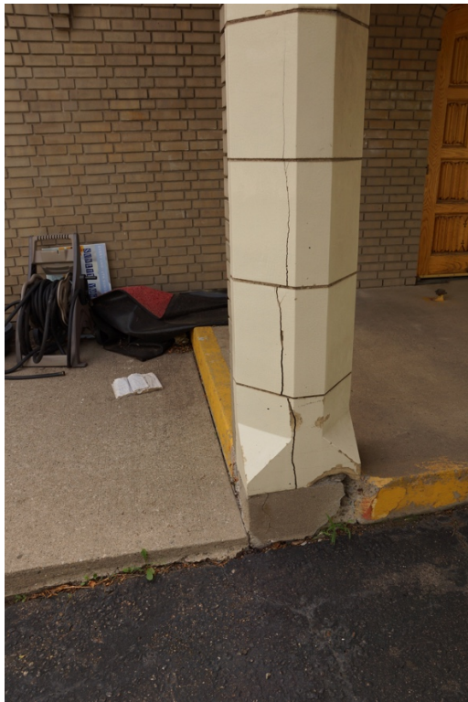
4048: Terra cotta damage
