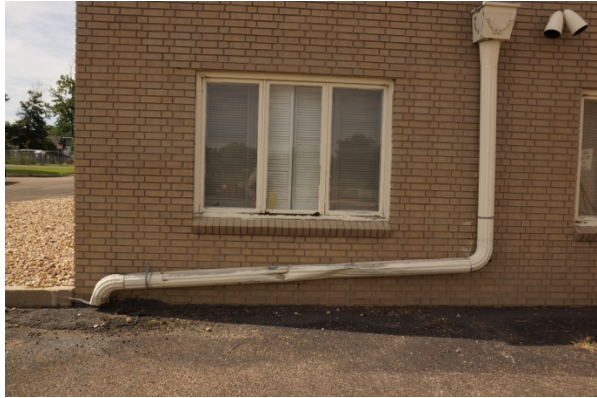
4032: Dented and dysfunctional roof drainage system components
