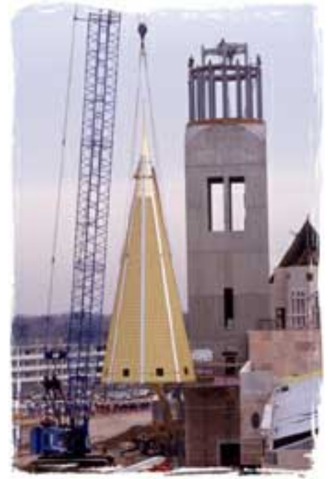
The Ritchie Center at the University of Denver — a grand, new building nears completion
