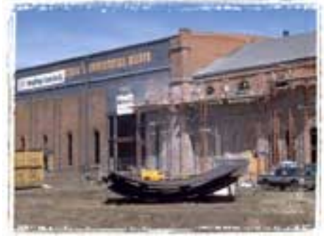
A historic trolley powerhouse is being converted to a new retail use for REI, a recreation outfitting company.
