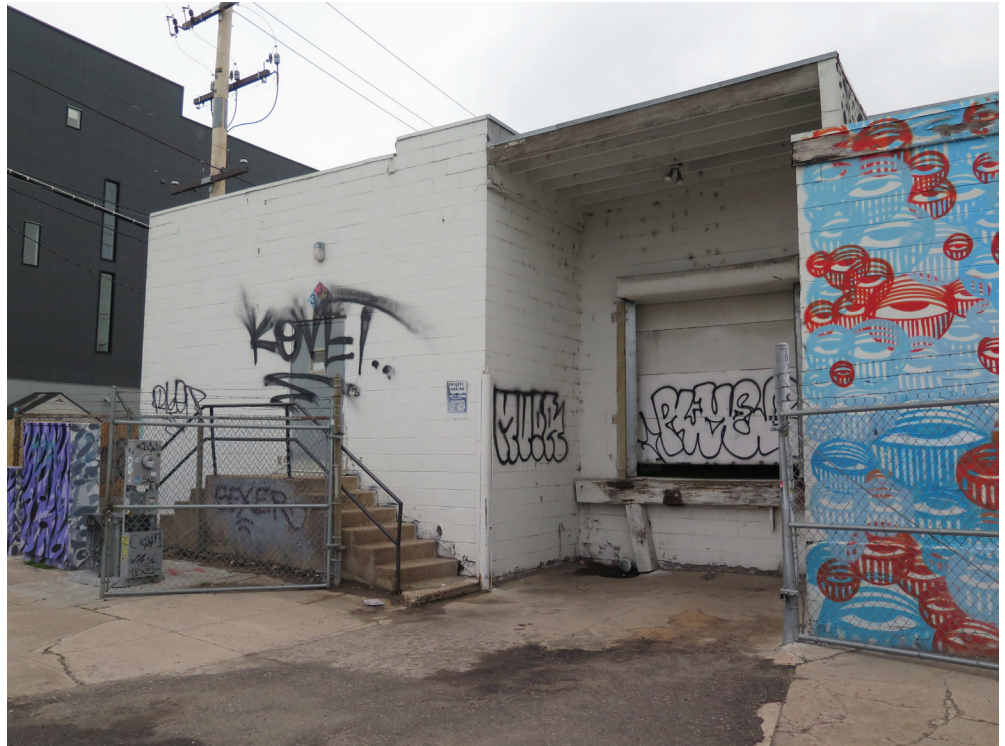
Deteriorated loading dock at the IMAC building
