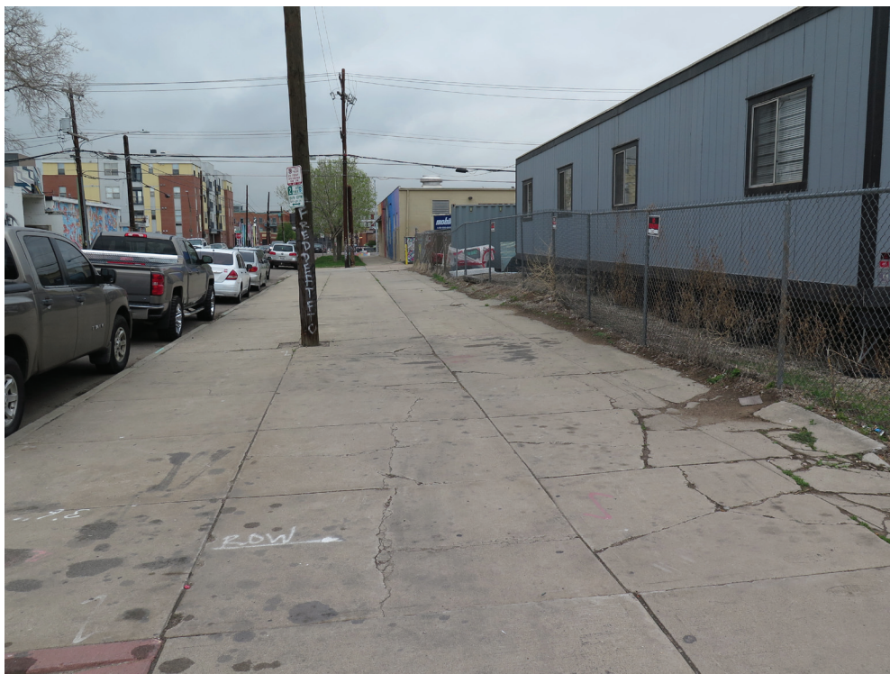
Lots of cracking in concrete sidewalk
