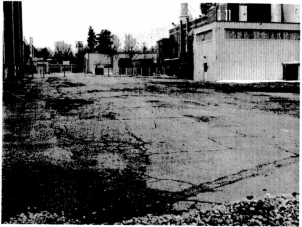
A large expanse of deteriorated pavement
