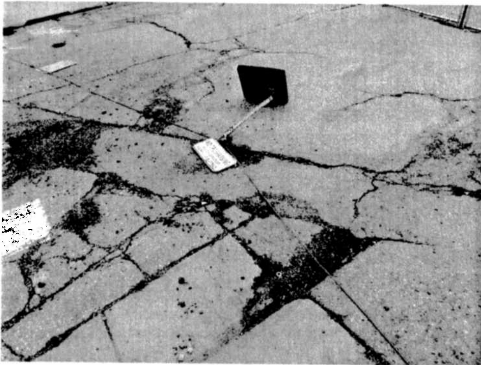
This deteriorated paved surface was typical of the condition of many parking areas in the Study Area
