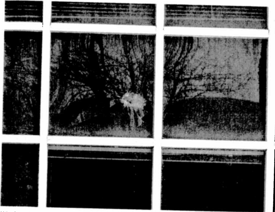
Windows broken by vandals were found in several locations
