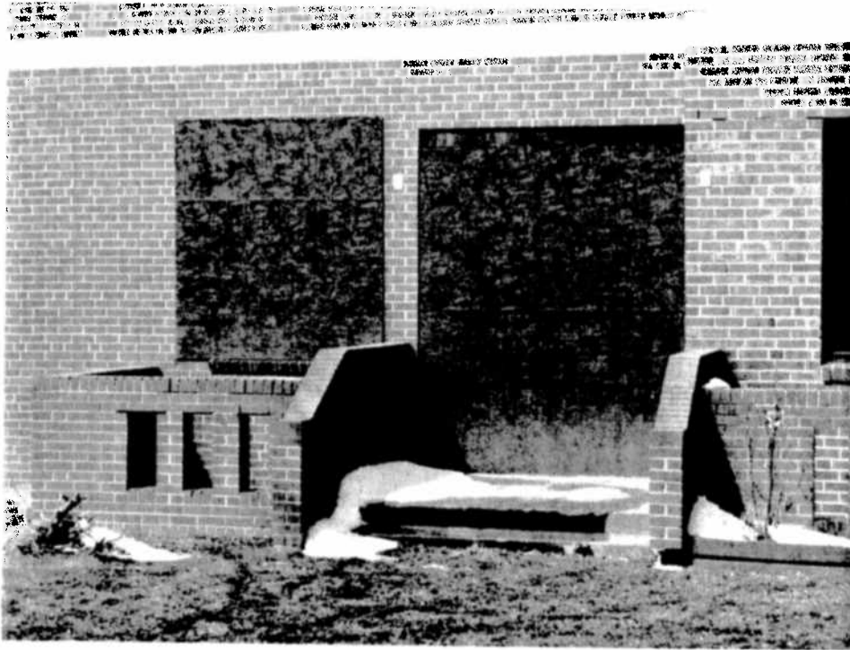
Boarded windows and doors were found throughout the Study Area
