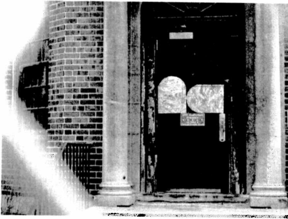
A door with broken glass panes and a deteriorated frame
