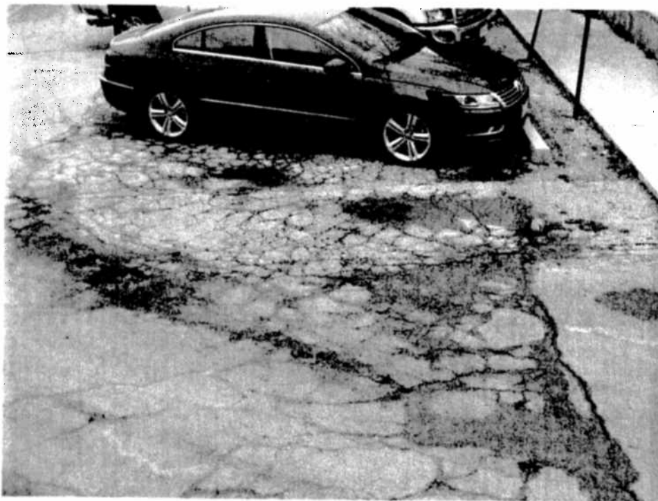
More crumbling pavement
