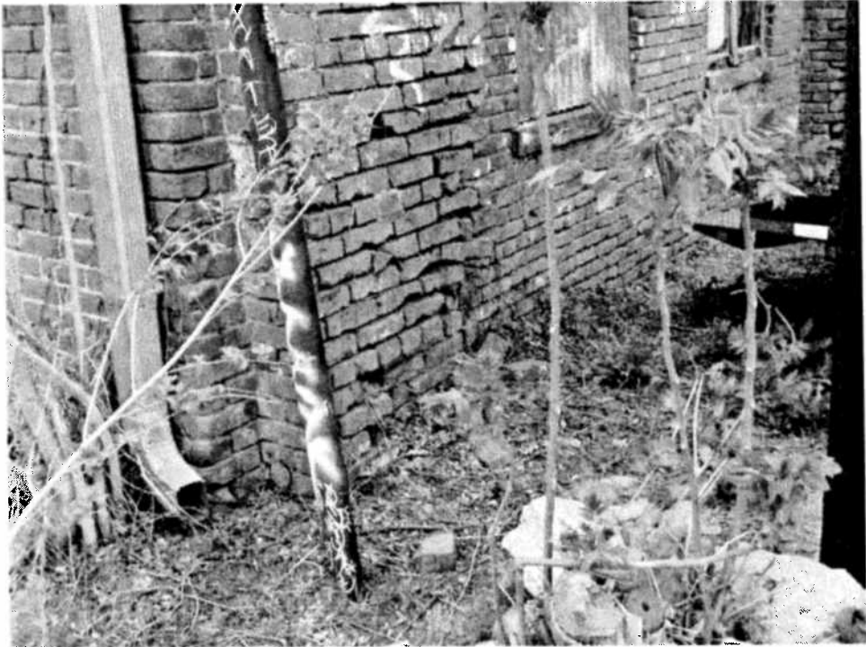
Exterior deterioration of the outer layer of brick
