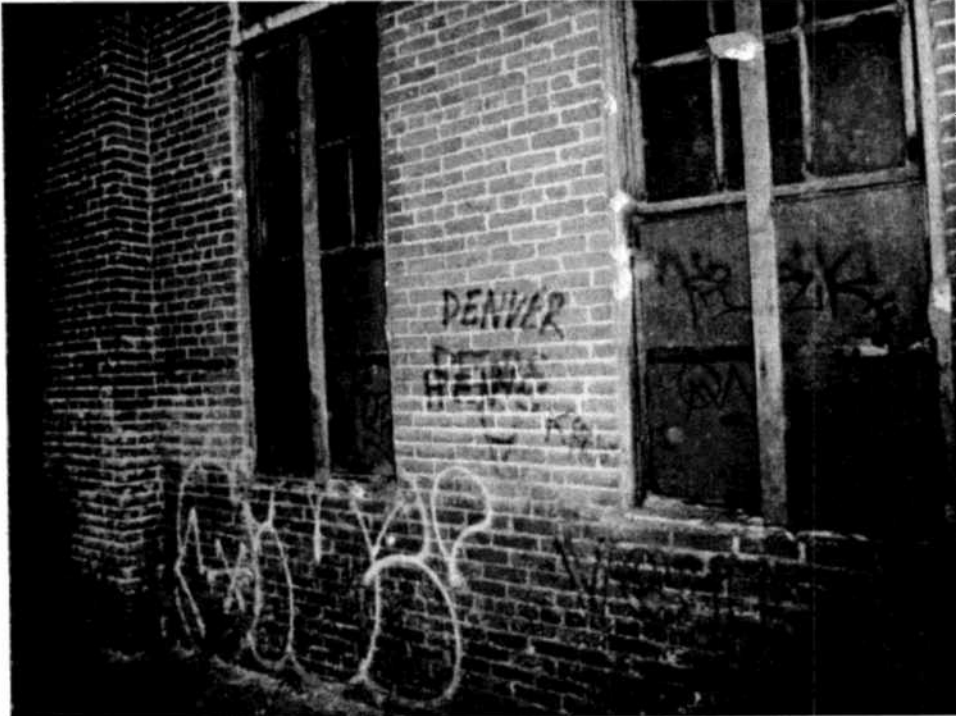
More boarded windows as seen from the interior
