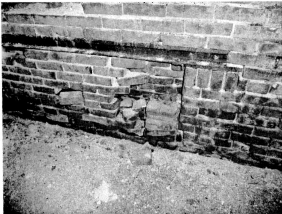
More crumbling brickwork could be found throughout the interior
