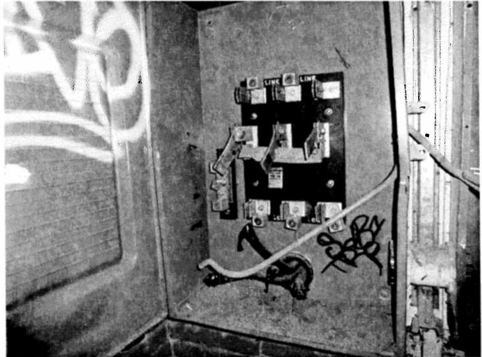
The building's electrical systems were no longer intact and would need to be brought up to code
