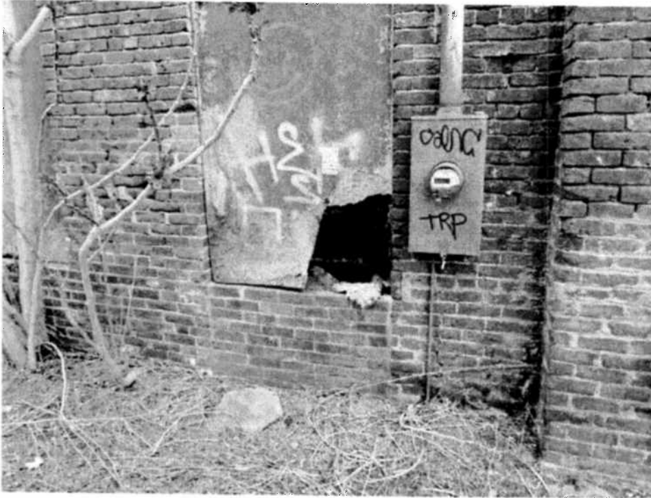
Another boarded window
