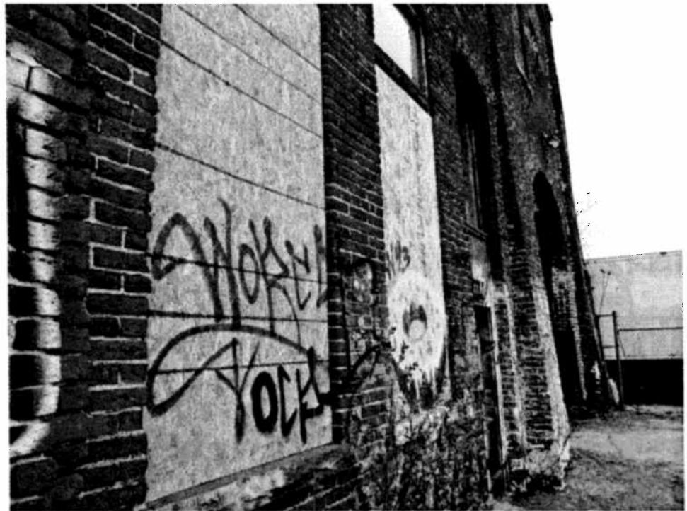
Many doors and windows were boarded up to prevent trespassing
