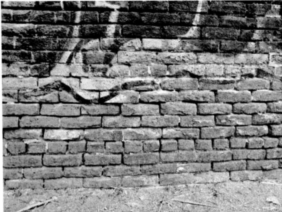
The exterior surfaces of the building were very deteriorated. Here, mortar is crumbling away from the brickwork, making the bricks loose and unstable
