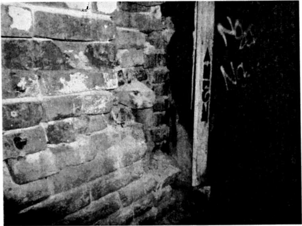
More crumbling brick
