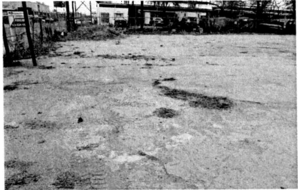
The concrete pavement throughout the Study Area was cracked, uneven, and deteriorated
