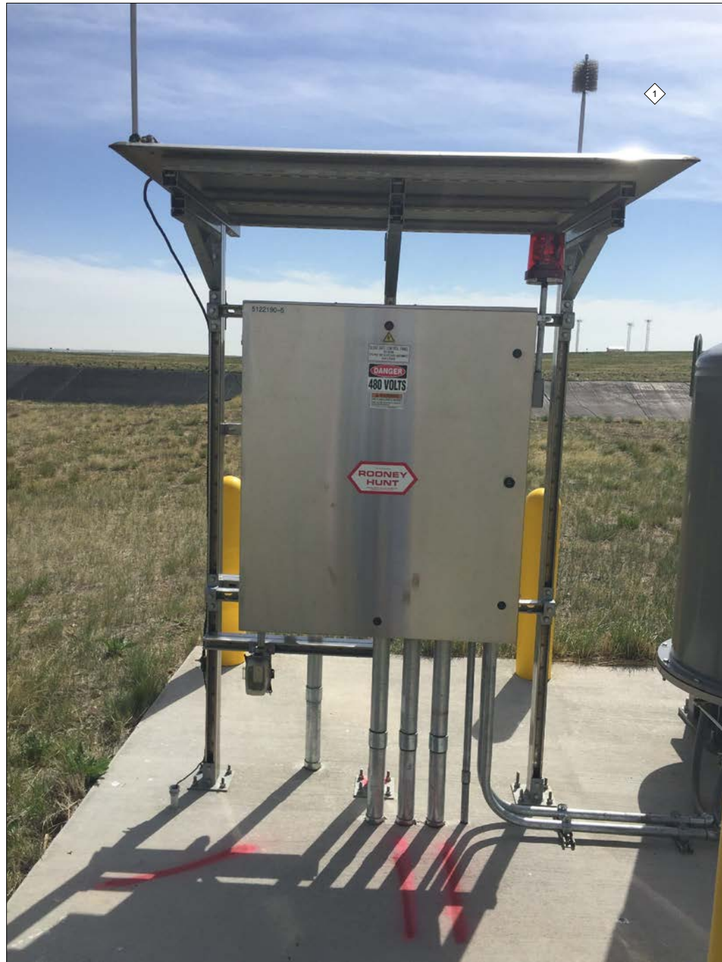
A1 EXISTING HYDRAULIC CONTROL PANEL E2000
