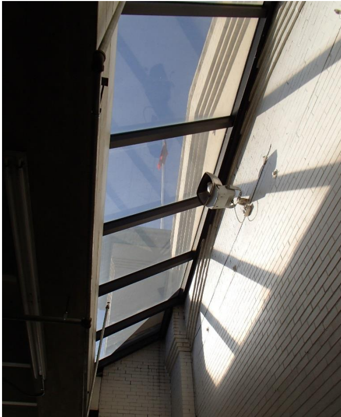
Figure 29. Skylight connection at the east upper-level interior door, showing the connection of Stadium Hall to Stadium Arena. Photographed February 9, 2016, Kathleen Corbett.
