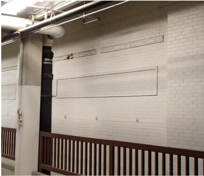
Figure 10. Infilled windows on the north side of the Stadium Arena, seen on the second floor of the Stadium Hall addition. The rusticated stone sills are part of the upper-level window, and the steel bar lintel extends across the tops of the infilled window openings of the lower-level windows. Facing southeast. Photographed February 9, 2016, Kathleen Corbett.
