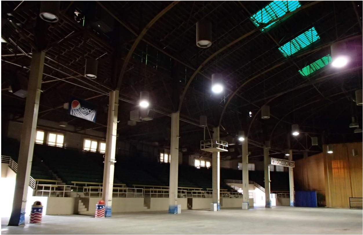
Figure 14. Interior of the Stadium Arena, showing the riveted steel columns. Photographed February 9, 2016, Kathleen Corbett.
