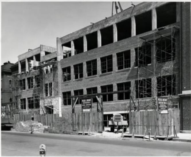
Photo showing construction of the first addition designed by Jamieson. This concrete-frame and brick clad addition was completed in 1947. Photo ca. 1946. Source: Denver Public Library
