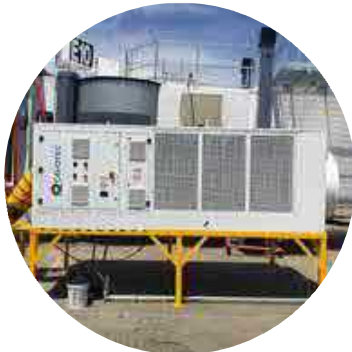
Ground mounted unit
