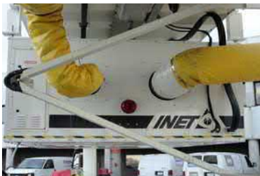
PCA hose connection at the AHU outlets
