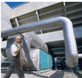
Air handling unit
