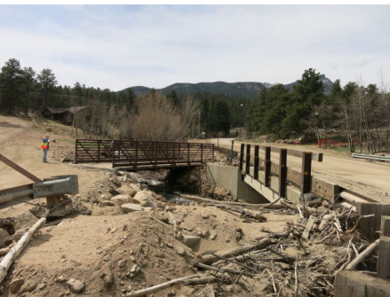
Damage from the Fish Creek Flood
