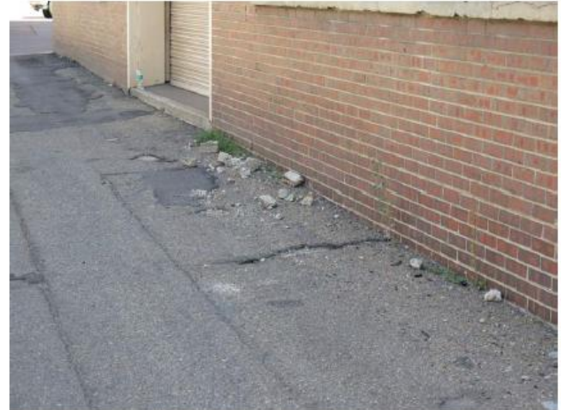
Chunks of concrete from the adjacent school building in an alley
