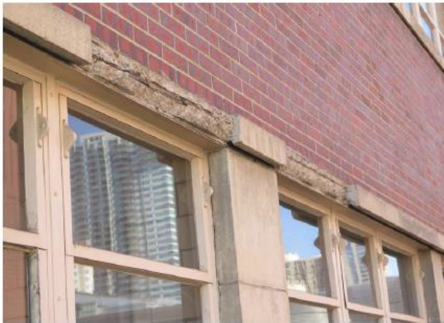
Deteriorated exterior elements above windows at Emily Griffith property
