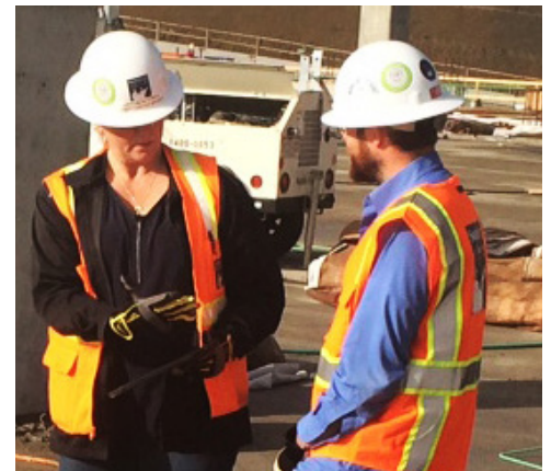
Christina Tetrick and Michael Brown perform quality inspection using BIM 360 Field at DEN
