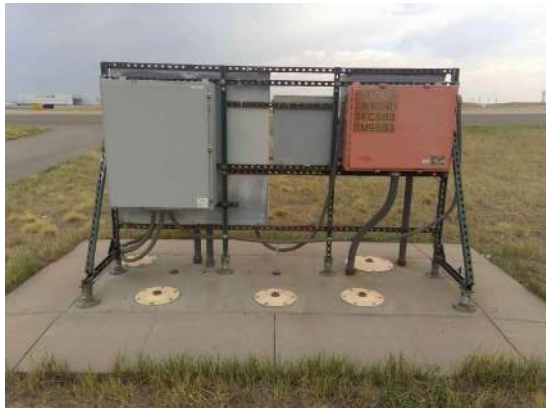
1 PHOTO OF RUNWAY 17R/35L RI/O (NORTH) - REMOVAL NOT TO SCALE
