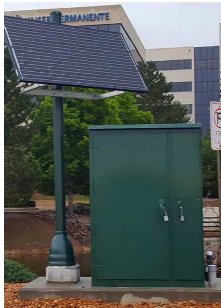
Figure 8 – Example above grade portion of a Flow Metering Manhole and Cabinet with solar power. Solar power is not required if utility power is available.
