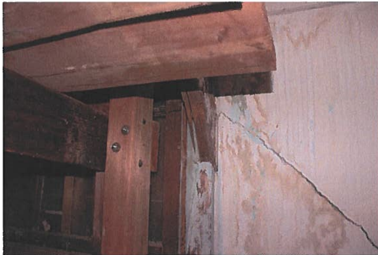
Figure Sixteen: Diagonal of a wood lateral frame in Building 1 the end of which is split
