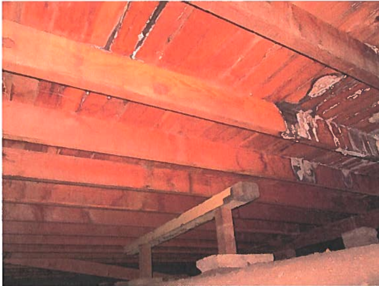
Figure Thirteen: Floor framing of Building 1. Note the joists, the tongue and groove decking, the intermediate bearing support, the lateral diagonal (beyond) and the posts below the center bearing line to the right of the image. Also note the stains on the decking and joists
