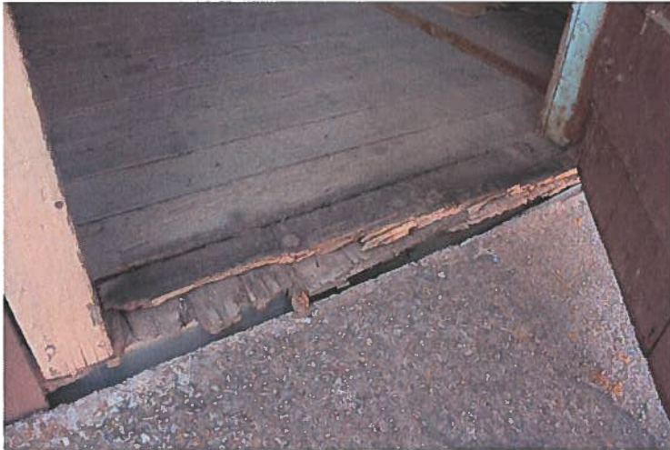
Figure Fifteen: Decay and wear of the subfloor and finish floor at west end of building at door sill
