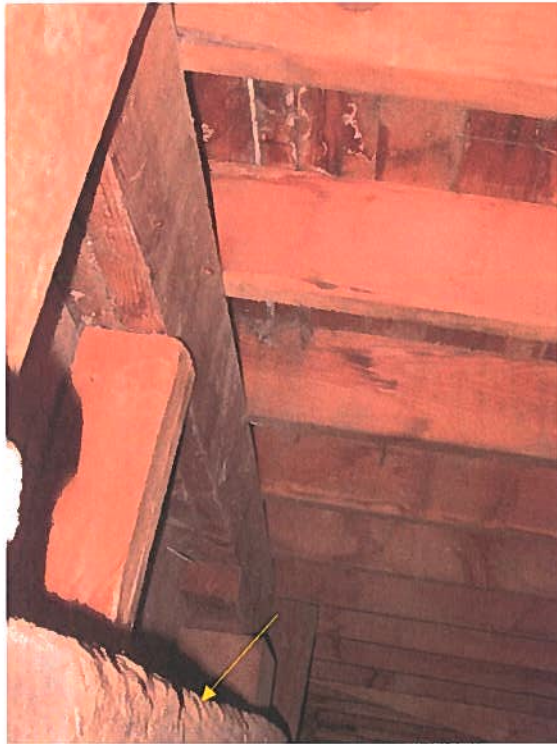
Figure Twelve: The double 2x6 beam supported on studs and posts. The posts and studs bear on a 7x7 plate visible at bottom of image.
