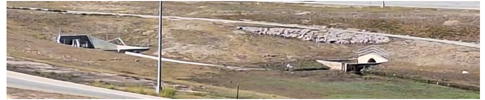
DEN Landside Stormwater System
