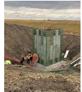
DS East (Phase 1) Storm Installation
