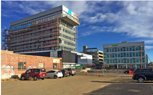
The Source Hotel (left) is currently under construction adjacent to the GreenBox mini-storage facility on Brighton Blvd. on the northwest side of the A Line commuter rail. This area would be included within both the DO-7 and IO-1 overlay districts.
