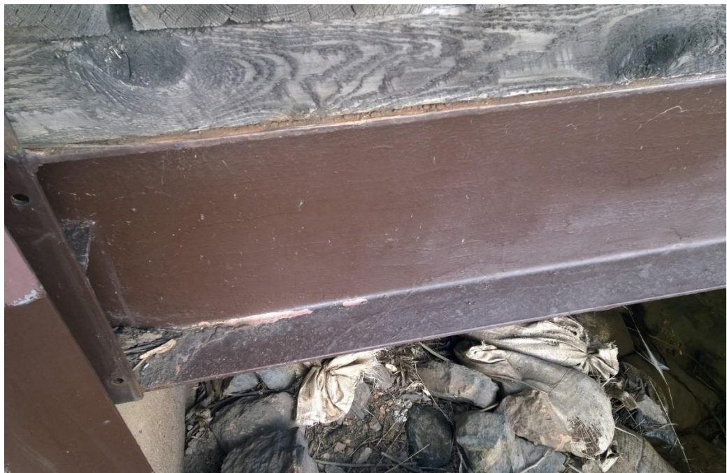
The dark brown paint (sample ELHB- PC01) on the metal substrate is not considered lead- based paint.
