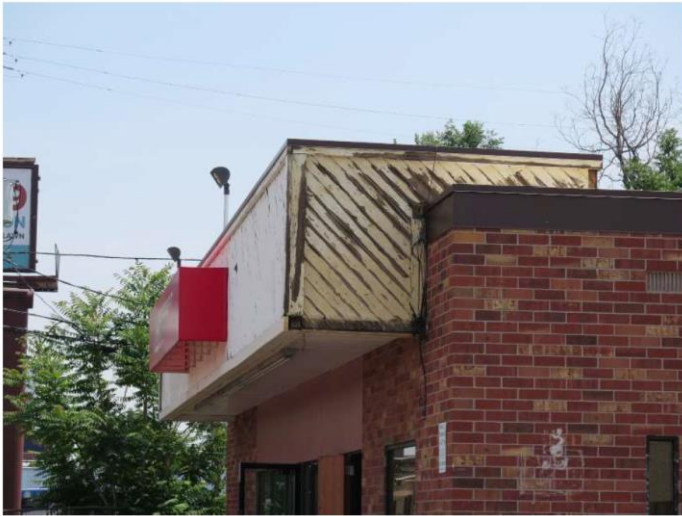
Retail building with peeling paint
