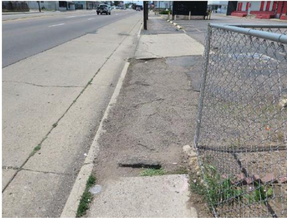
Sections of damaged asphalt in public sidewalk right-of-way along Colfax
