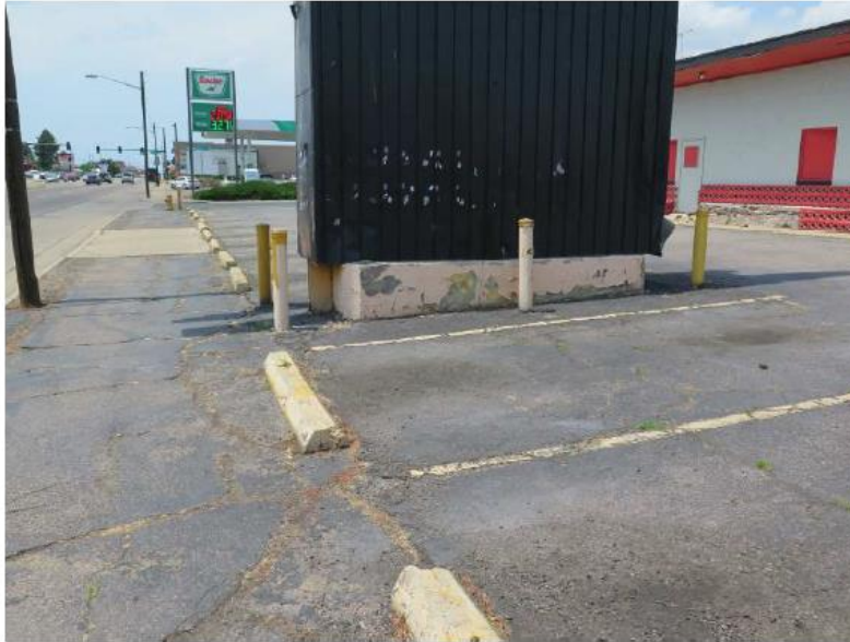
A dilapidated sign on with deteriorating asphalt serving as the public sidewalk
