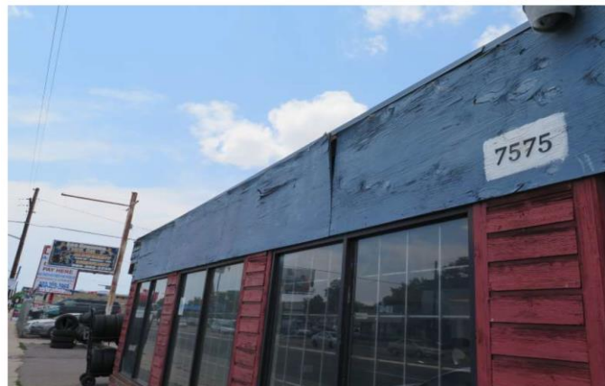
Deteriorated exterior surfaces
