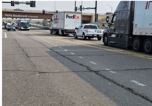
Pavement conditions, Jackson Gap
