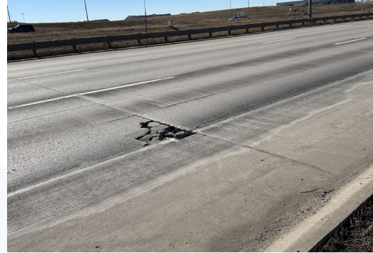
Pavement conditions, Peña Blvd.
