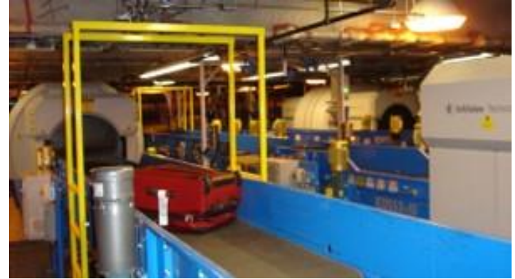
DEN's Existing EDS Equipment
