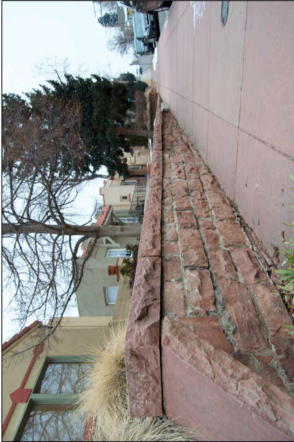
Looking northeast at sandstone wall along southern property boundaries (119 closest on the left)
