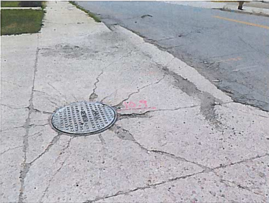
Degraded concrete curb cut at the Xcel-owned facility
