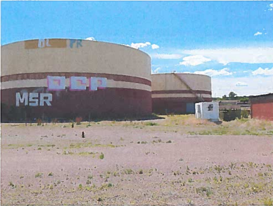
Graffiti on the storage tanks
