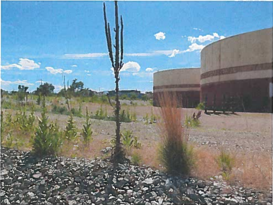
Tall weeds on the storage tank site
