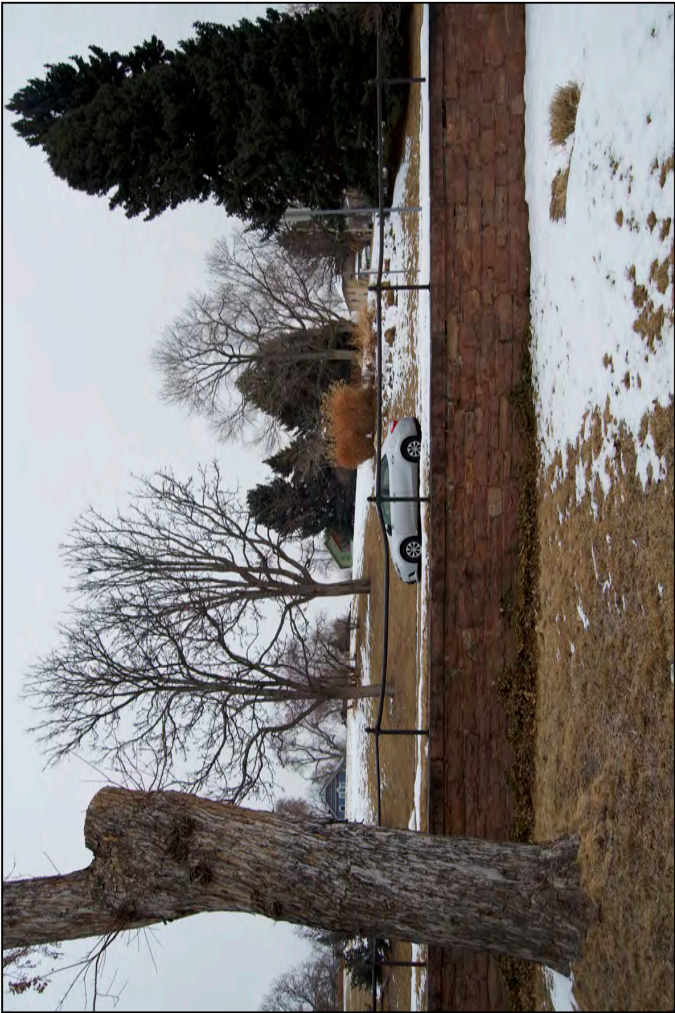
Looking east from sunken backyard of 141 E. Vassar Ave. at stone wall and metal railing
