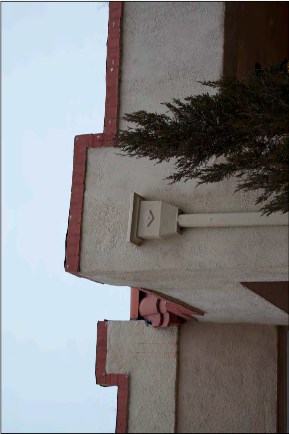
Original downspout and closeup of parapet with brick coping on 135 E. Vassar Ave.
