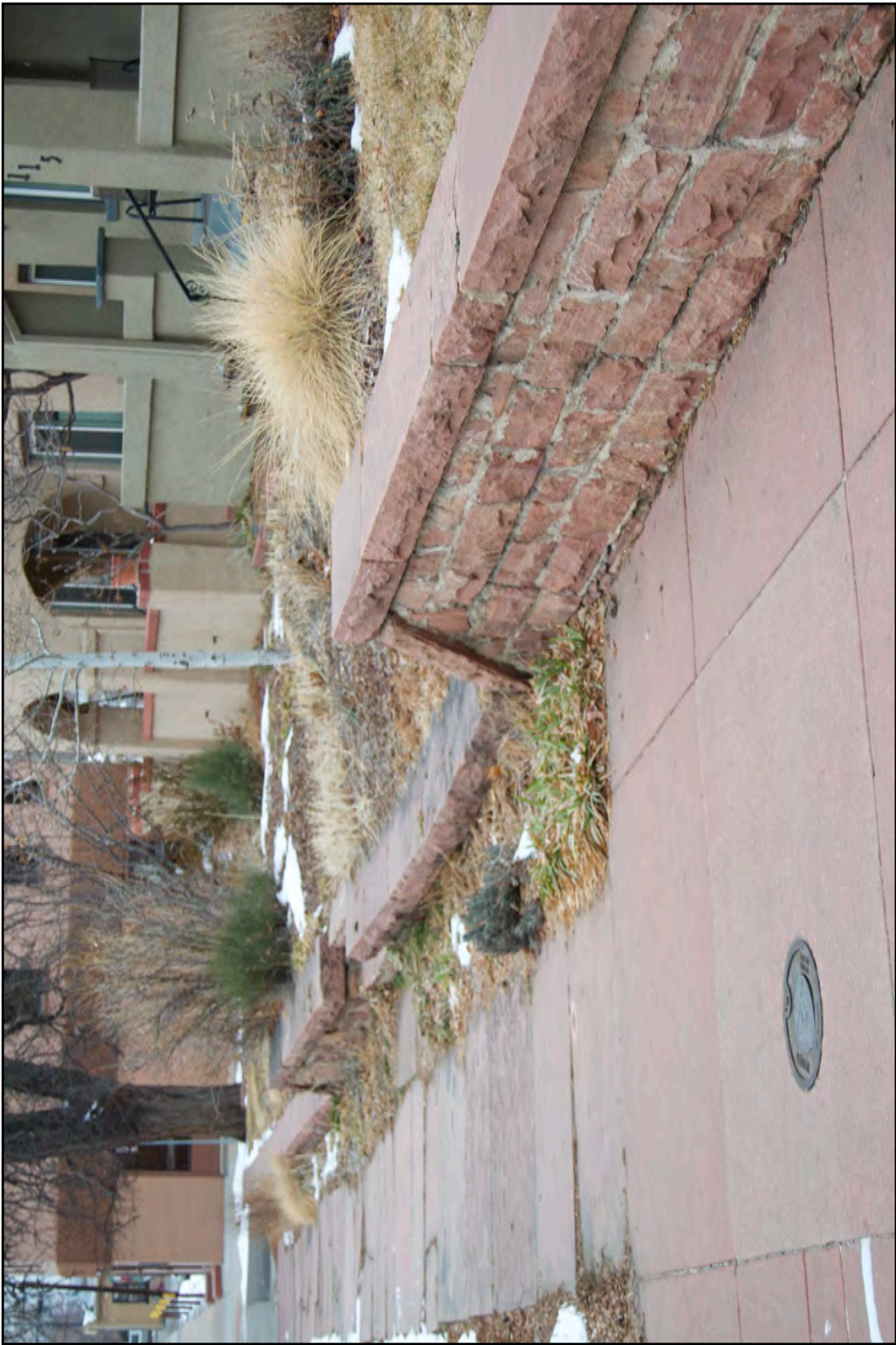
Looking northwest at sandstone wall along southern property boundaries (15 closest on the right)
