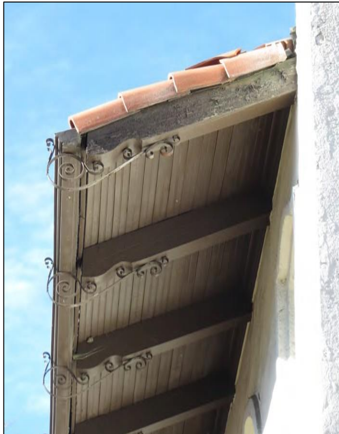
Photograph 4 (right): South side close-up of overhanging eaves with shaped rafter tails, iron scrollwork, and red tile roof
