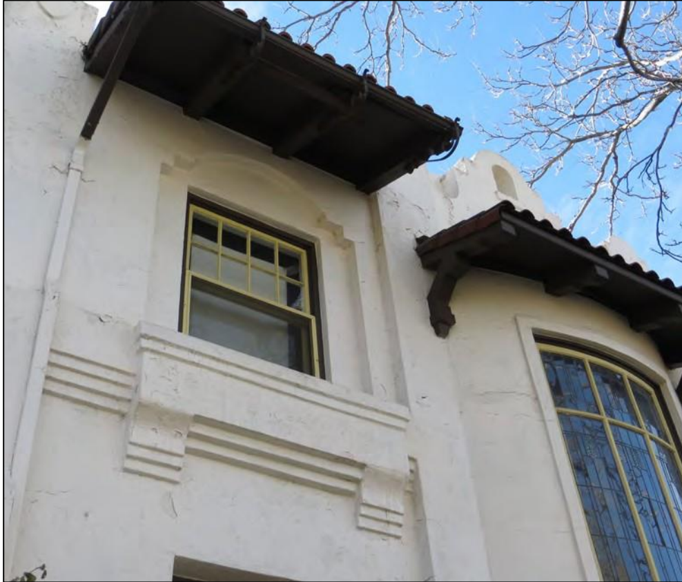
Photograph 5 (left): North side close-up of overhanging eaves, pent roof, and bow window
