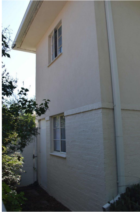
20. North wall of the 1949 addition. Photographer: Thomas H. Simmons. Date: August 2022. View east-southeast.
