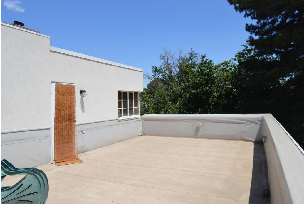
14. Second story and roof terrace from southwest corner of the terrace. Photographer: Thomas H. Simmons. Date: July 2022. View east-northeast.
