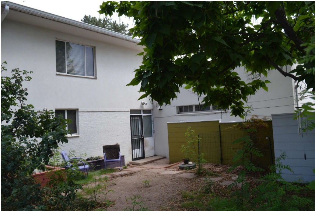
22. West of the 1949 addition and north wall of the garage. Photographer: Thomas H. Simmons. Date: July 2022. View southeast.
