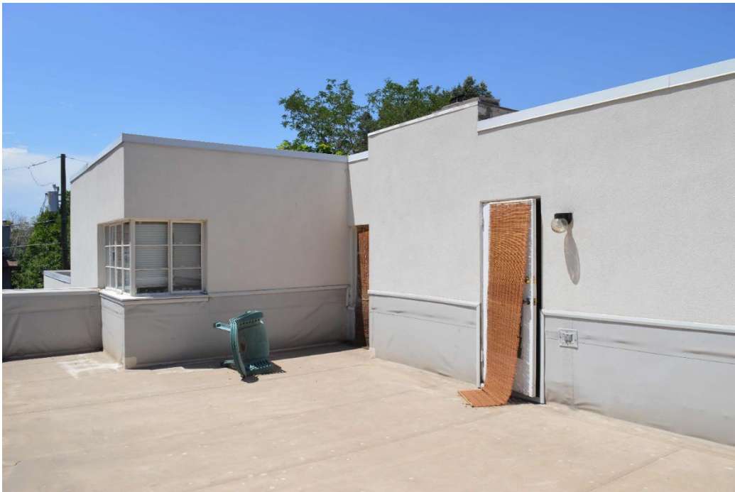
13. Second story and roof terrace from southeast corner of the terrace. Photographer: Thomas H. Simmons. Date: July 2022. View west-northwest.
