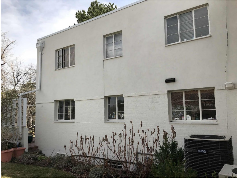
18. North wall of the house east of the 1949 addition. Photographer: Linda McVey. Date: April 2019. View southeast.
