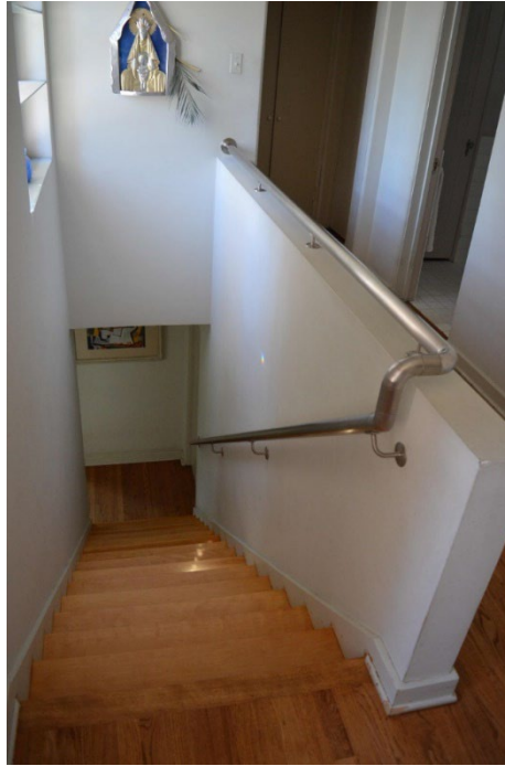
28. Interior, second story, stairs and second story stair hall, showing fluid railing detail. Photographer: Thomas H. Simmons. Date: July 2022. View west.
