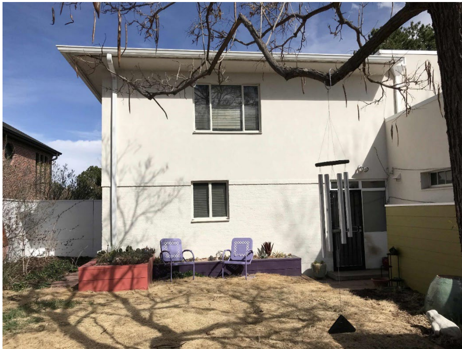
21. West wall of the 1949 addition. Photographer: Linda McVey. Date: April 2019. View east.
